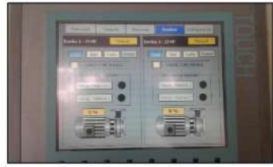
HMI – PANTALLA BOMBAS
