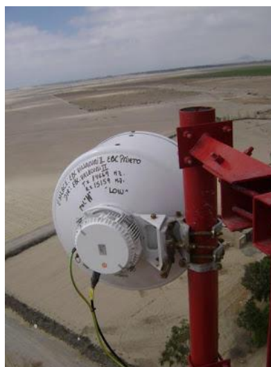
Figura 31: Antena MW Huawei - EBT Villacuri Ica
