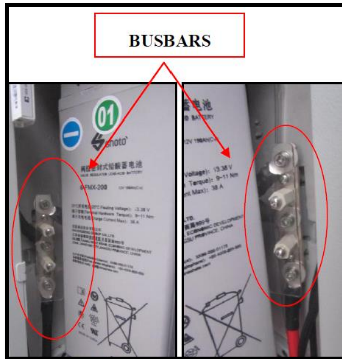
FIGURA 3-41: BUSBARS, Site Santa Teresa
