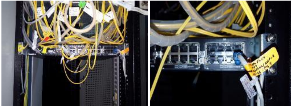
Figura 39 - Router Tellabs 8609 – Central Huaraz.
